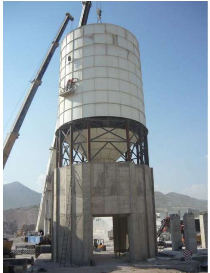
Figure 5: 1,000 ton capacity silo. This particular silo, manufactured by Zimmerman Industries, is 70 ft. tall, 27 ft. in diameter, and weighs 8 tons.
