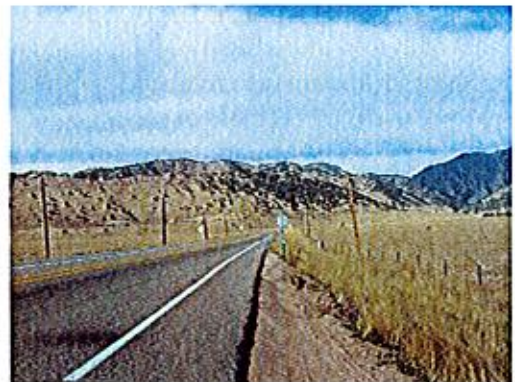
At MP 10.5, SH-72 traverses the base of the foothills west of the SH-93 intersection.
